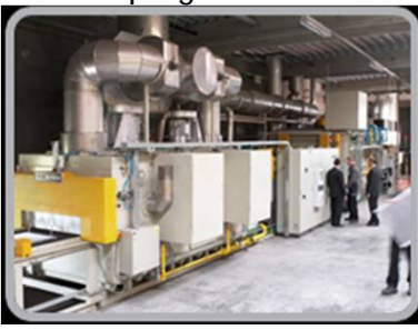
Refrigeration Rack System
